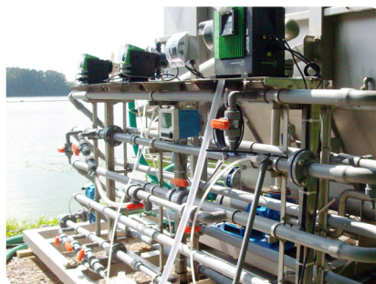
Chemical feed pumps dose coagulant and flocculant into the flocculator.
