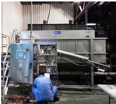
Electric and pneumatic control panels automate DAF system operation.
